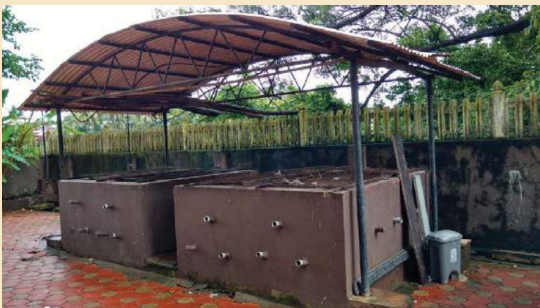
Photo 7.8c Decentralized Composting Units in Panaji, India
